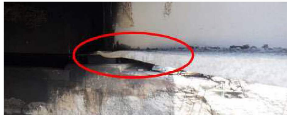
Bottom flange lateral and vertical distortion
