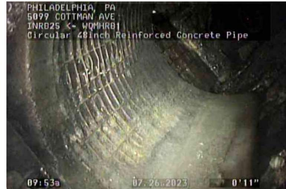
Damaged Concrete Pipe
