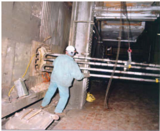
Corrosion and Coatings Investigation
