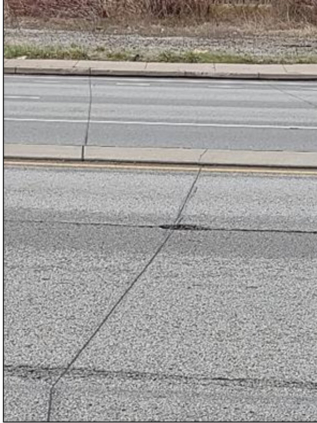
Figure 29: Route 51 Partial Depth Repair with Overlay Failure
