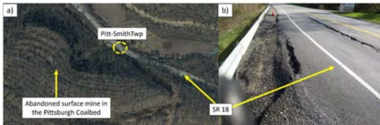
Figure 4.7.13. a) Pitt-SmithTwp landslide occurred along SR 18 from Google Earth. The top of the image is oriented to the north.; b) uneven pavement, large cracks, and asphalt sinkholes.
