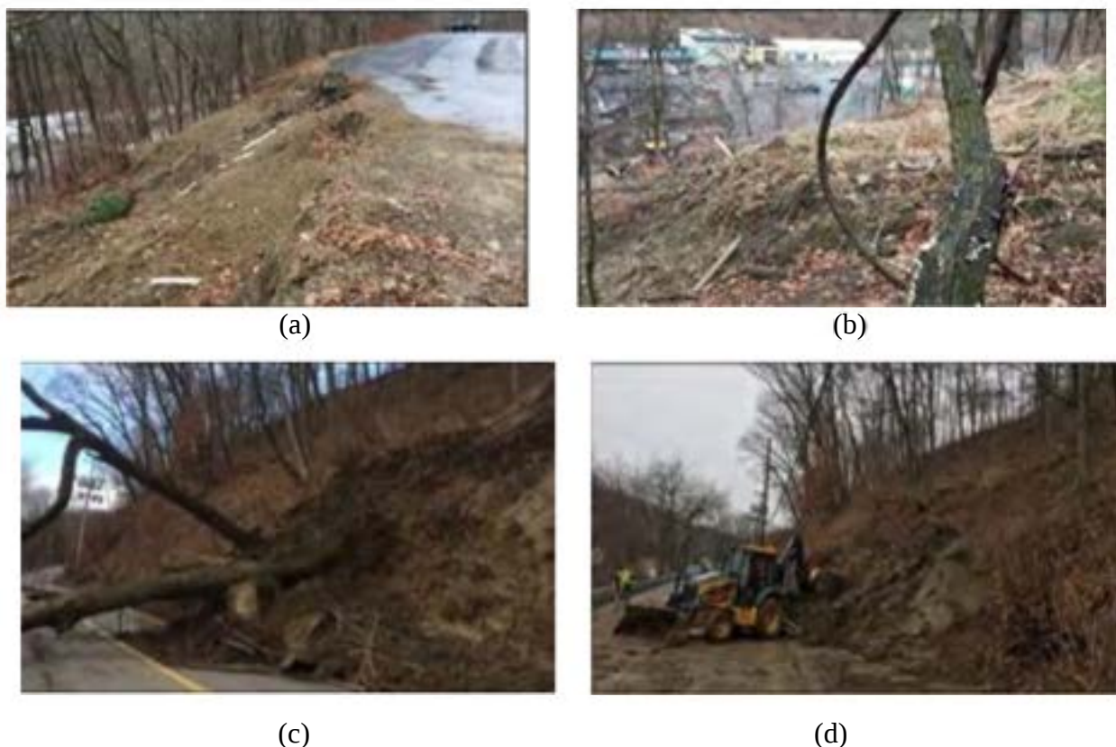
Figure 4.6.2. Pictures of the Evergreen road slides (from (DöAppolonia Engineering, 2018a). Panel a) upper limit of the landslide at Evergreen Road from Rico's Parking Lot -- looking west; b) landslide debris on slope at Evergreen Road -- looking south; c) Landslide debris on Evergreen Road -- looking west; and d) clearing of landslide debris from Evergreen Road -- looking west (DöAppolonia Engineering, 2018a).
