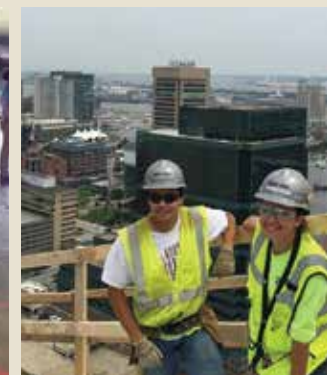
Nicole Yanouzas (Civil) (right), and a fellow co-op work on roof construction with Baker DC in Baltimore, Md.
